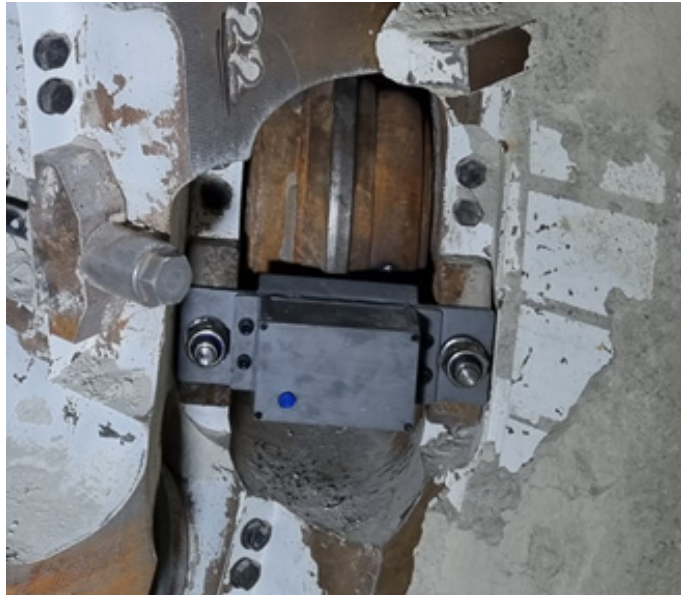
Fig. 17. Installed a wear sensor package on disc cutter No.22
